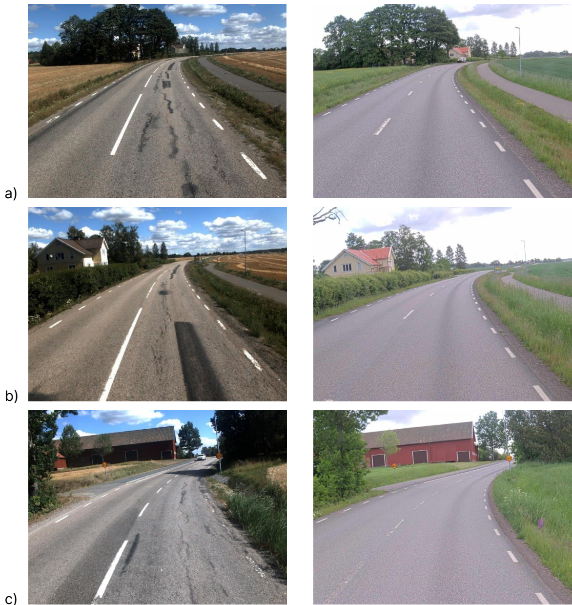
Figure 2. Photos from road 190 in three different locations. The road is in poor condition with severe cracking, alligator cracking and large rut depths. Photos taken in 2018 before the maintenance work are shown in the left column and the most recent photos, taken in 2022, are shown to the right. Photos: Trafikverket, PMSv4.
